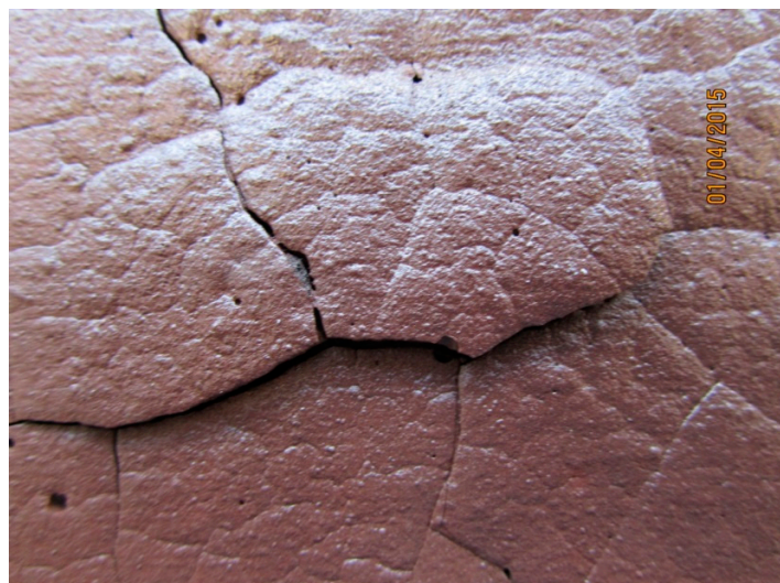
Figure 10. C1.82PP hot side close up showing lifting section attributed to differential thermal expansion/delamination. Healing of other cracks is also evident. Note that this region is clearly visible in Figure 9b and has been enlarged 1.5×.
