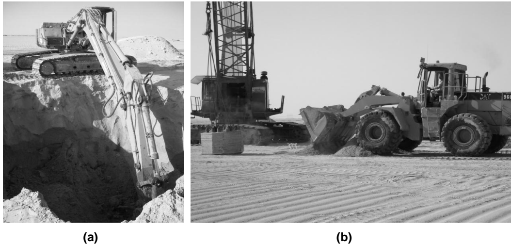
Figure 3. (a) Pre-excitation, (b) backfilling with sand and compacting with a heavy poulder
