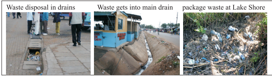
Figure 2: Eroded earthen roads and trenches at some of the beaches
