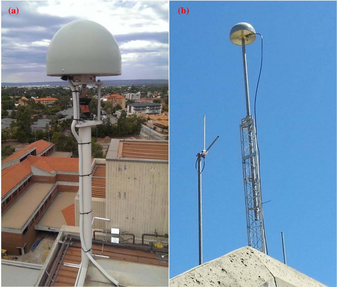
Fig. S1 Setup of CUT00 (subplot a) and SPA00 (subplot b): the distance between two antennas is about 358 m.
