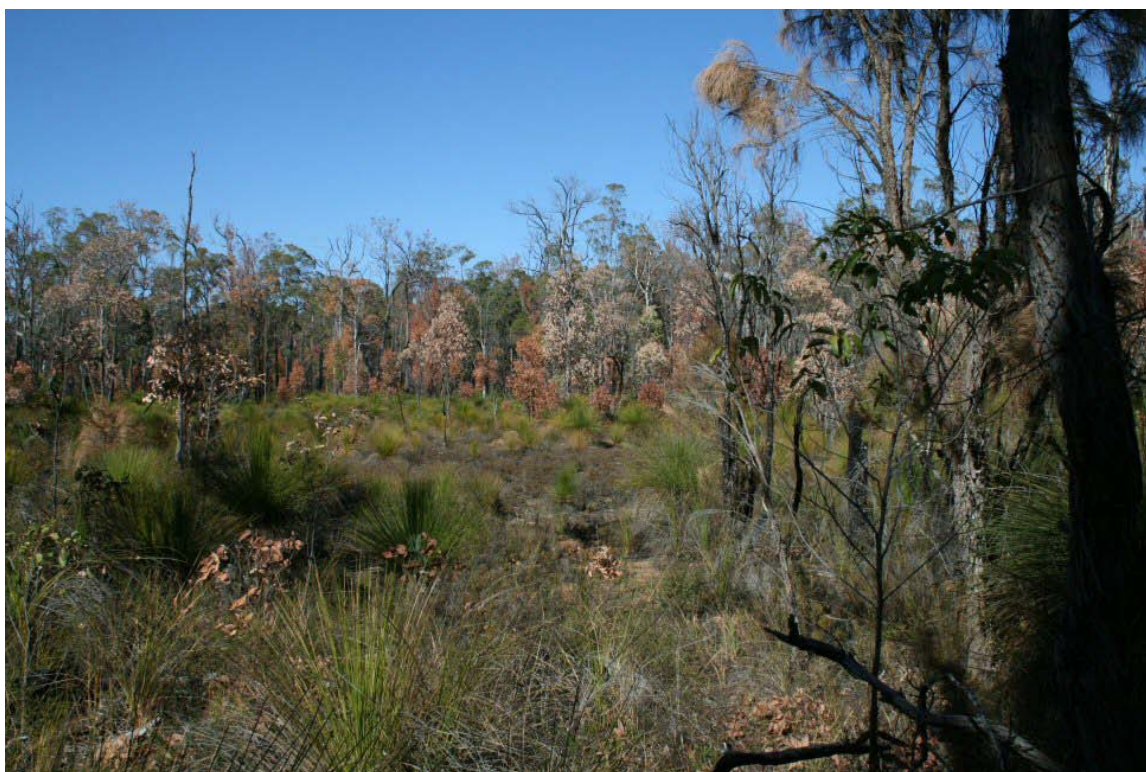
Figure 12. Site N1. Recently dead trees around a rocky outcrop which is close to the surface.
