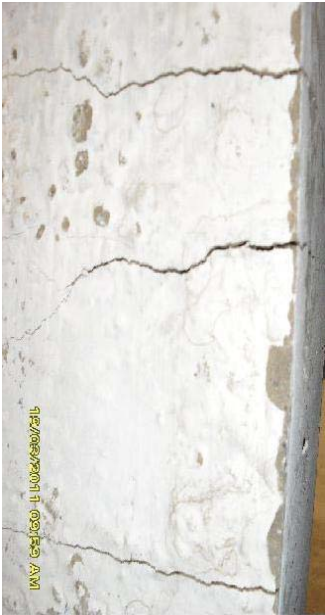
(a) Cracks on tension sides
