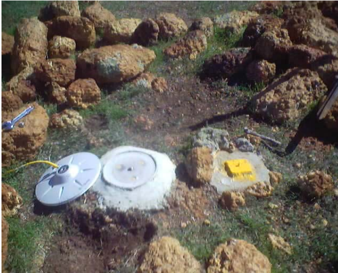
Figure 2. A newly installed ground monument (left); the ground mark to the right is part of the existing Western Australian geodetic network maintained by DLL.
