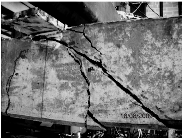
Figure 6. Typical shear compression failure
