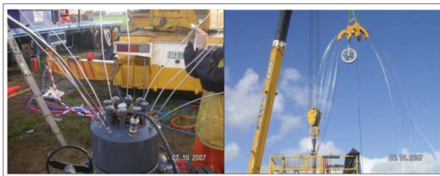
Figure 5. Assembling and deployment of the complete system was a complex and successful operation. These figures show the wellhead with flow tubes and cable connections (left) and control of the u-tubes while inserting the integrated assembly (right).
