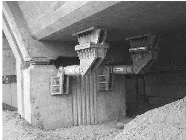
Figure 12. Shock transmission unit installed in a bridge.
