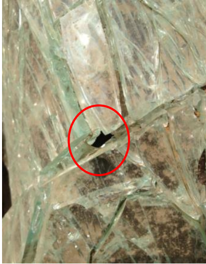
Figure 15 PVB rupture observed on pane 1-1-1
