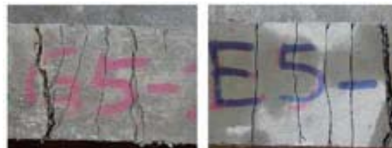
Figure. 8: Multiple Cracking Patterns in DFRGC (Left, PVA-1; right, ST+PVA-1)
