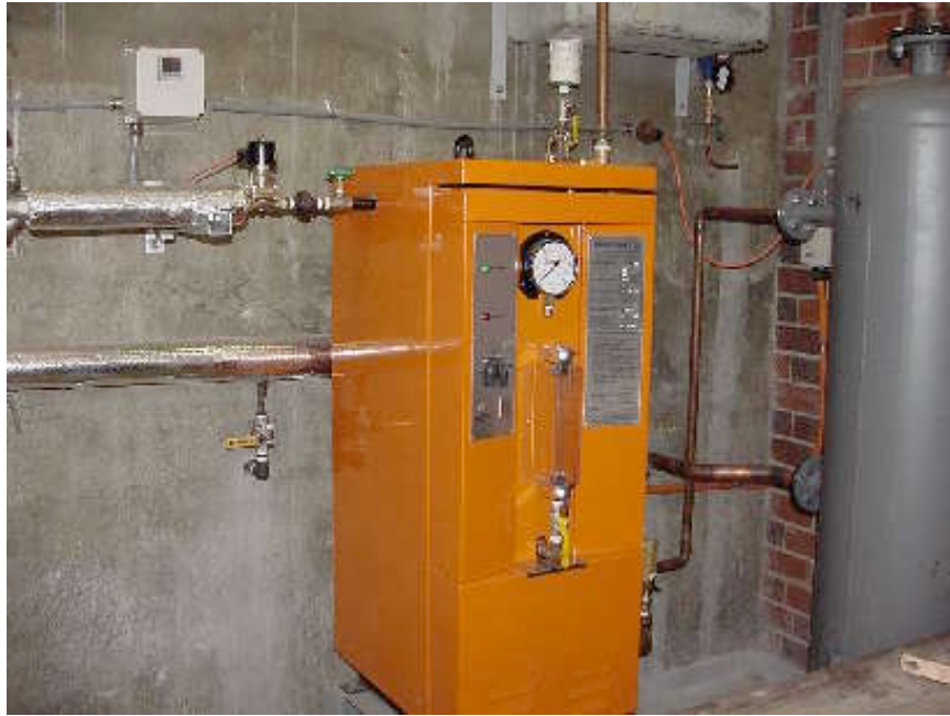
Figure 3.13: Steam Boiler and Controls
