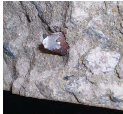
(b) Typical Fracture of Mesh Bars Observed
