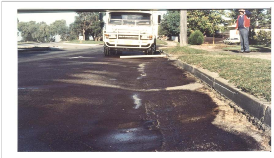
Figure 2.4 - Rut Failure (Nicholson Road WA, Picture is provided by Colin Leek)
