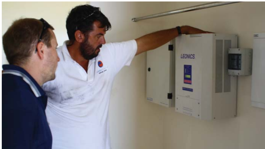
Figure 7-26 : Distributed Villa Inverters
