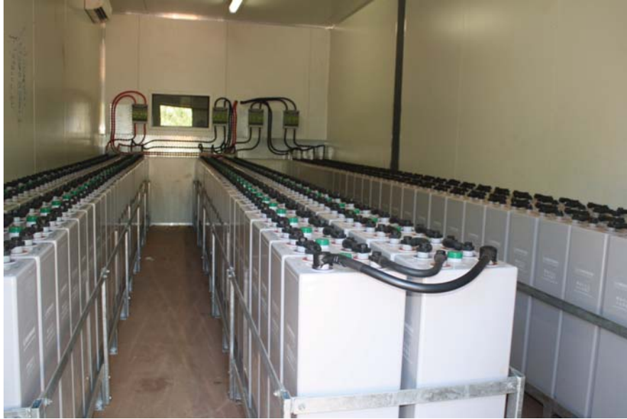
Figure 7-24 : 360V 540kWh battery room installation
