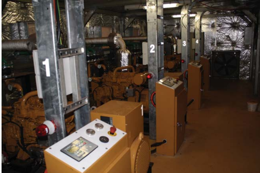
Figure 7-29 : 4 x 50kVA Hino diesel generation plant
