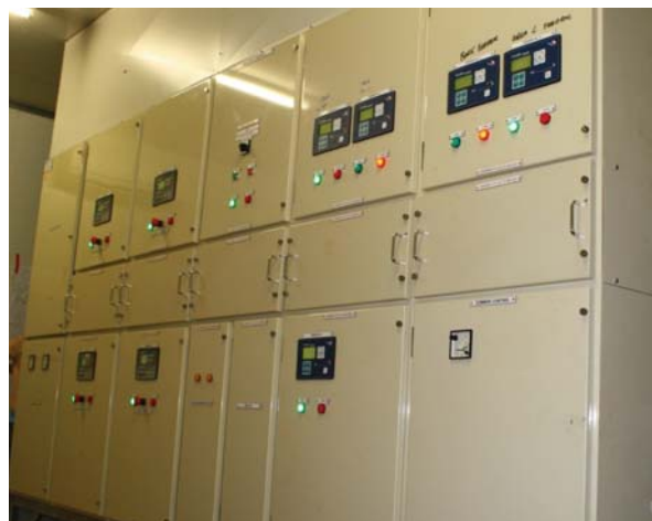
Figure 7-28 : Powerhouse main switchboard
