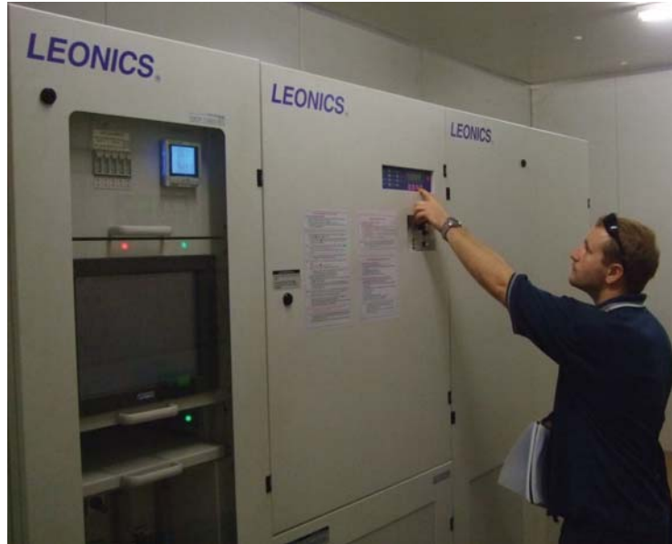
Figure 7-27 : Central inverter and controller
