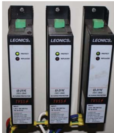
Figure 7-30 : Lightning protection at main switchboard
