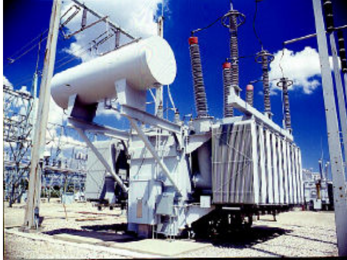
Figure 1-1 Power transformer, front view
