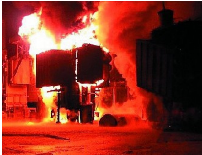
Figure 1-2: Picture of transformer explosion
