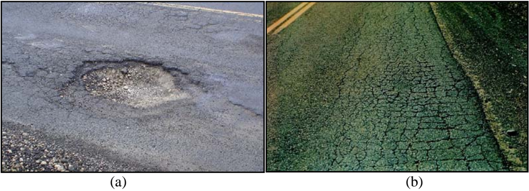
Figure 2: Deteriorated pavements due to Water induced damage, (a) pothole (b) alligator cracking (pavementinteractive.org)
