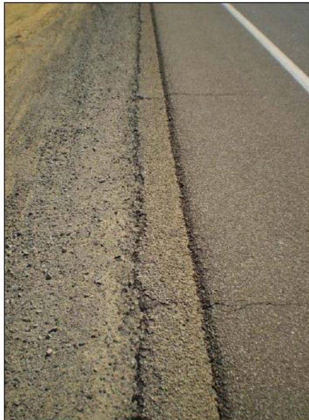
Figure 2.6: Transverse cracking of trial pavements with HCTCRB basecourse (Harris and Lockwood 2009)
