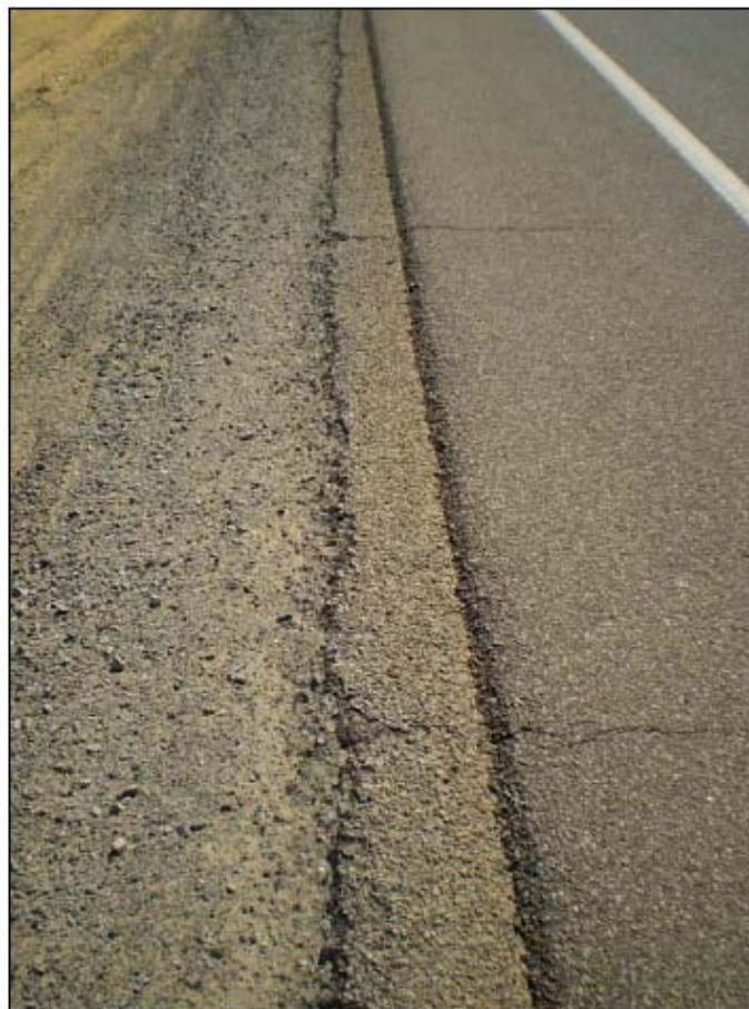
Figure 3: Transverse Cracking of Trial Pavements with HCTCRB Base Course
