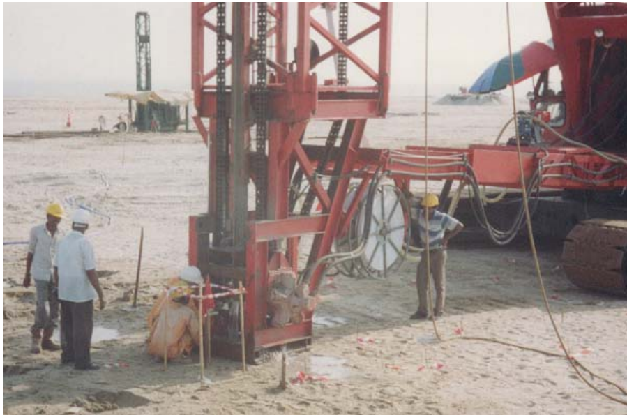
Figure 5.5 Close-up of vertical drain installation works (note roll of drain material which is threaded through mandrel).
