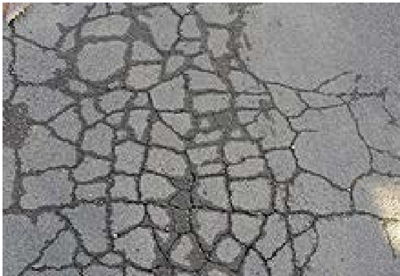
Figure 2-1 Typical Fatigue (Crocodile) Cracking
