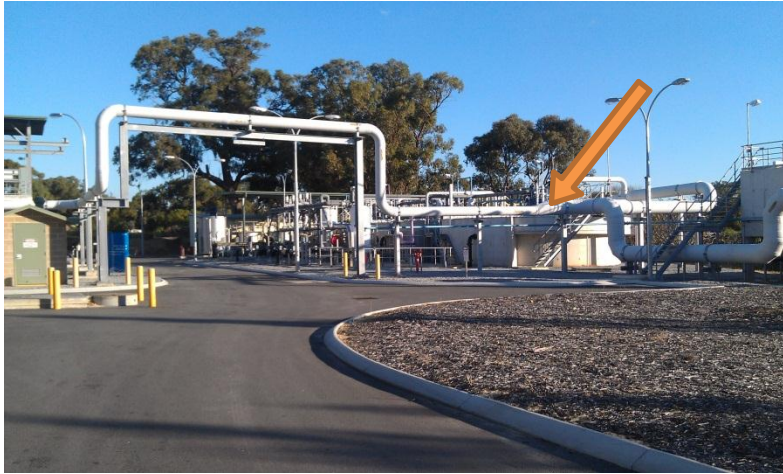
Figure 3.4: Thickened activated sludge sampling point at the DAFT units
