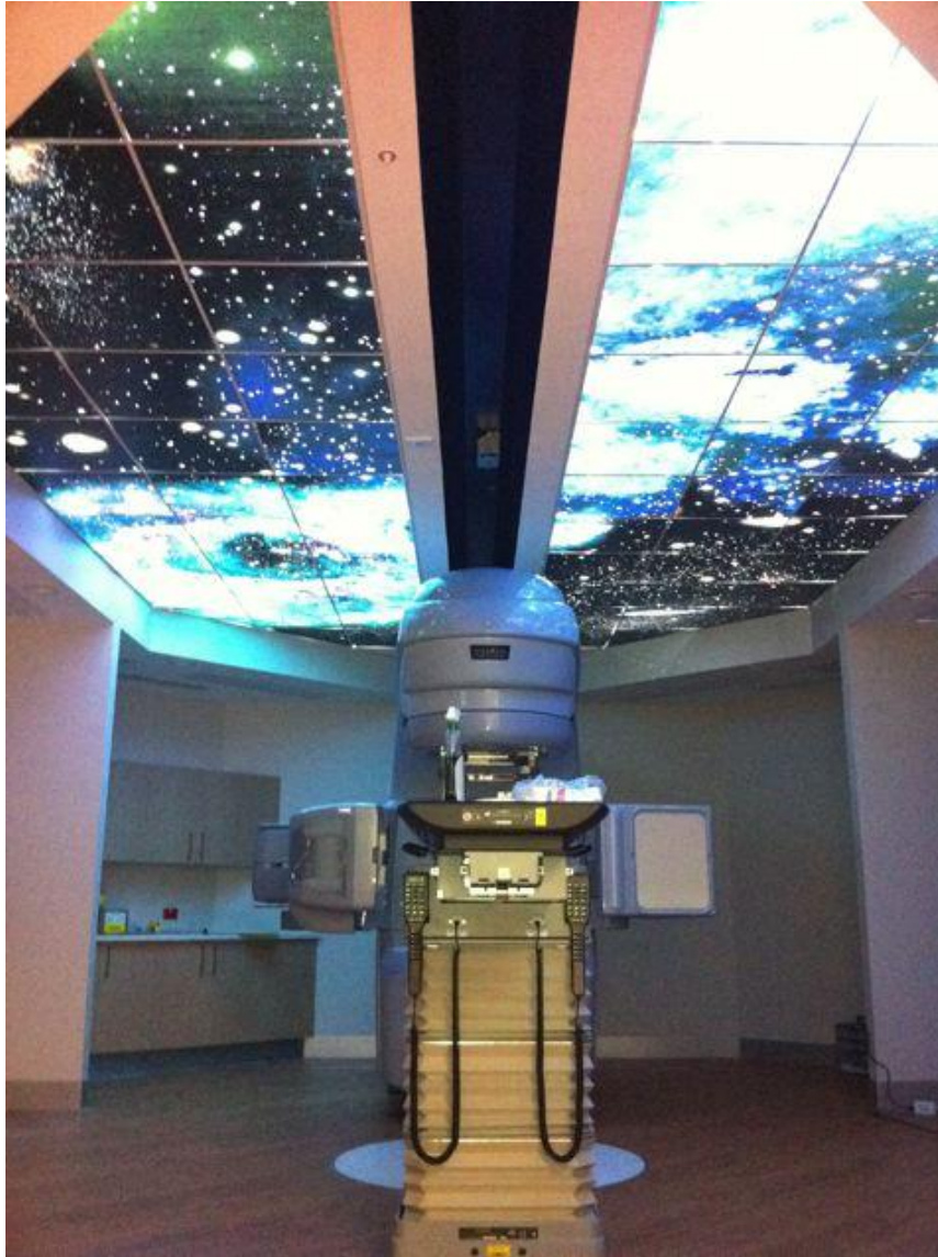
Figure 13 One of the treatment bunkers, Sunshine PMac centre, showing the position of linear accelerator and the night ceiling effect. (Courtesy of B. Taylor, Peter MacCallum Cancer Centre, 2011)
