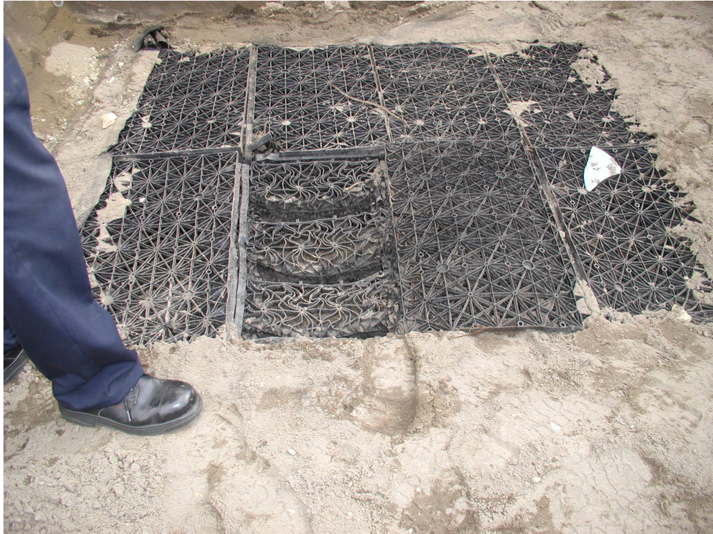
Figure 3: Collapsed Plastic Grid System (courtesy of City of Canning)
