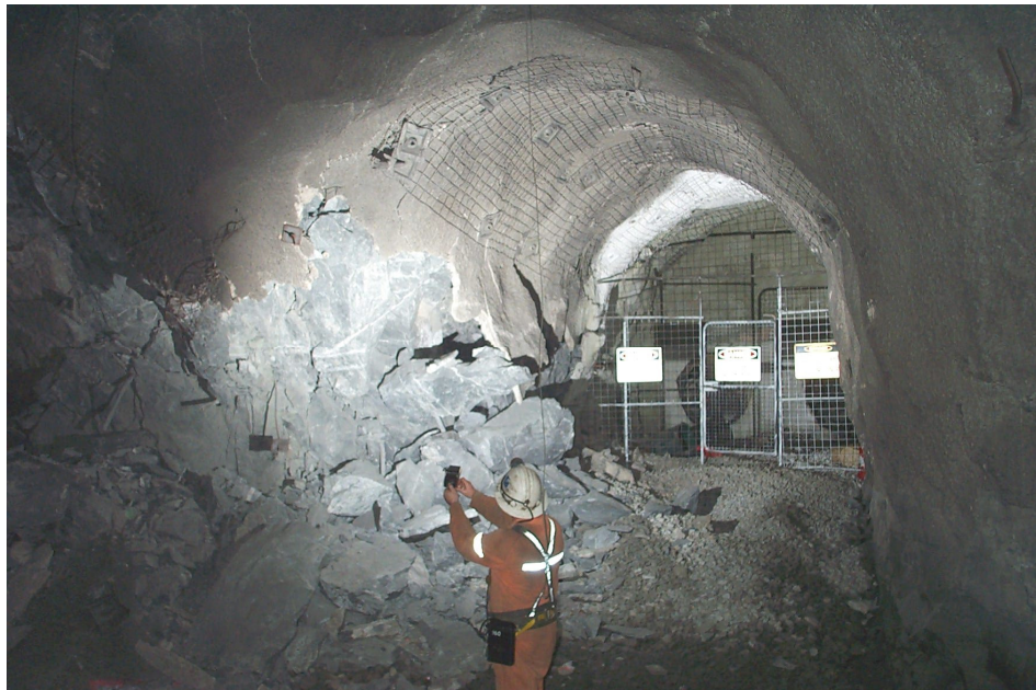
Figure 2.18 Rock burst causing failure of the installed support in sidewall
