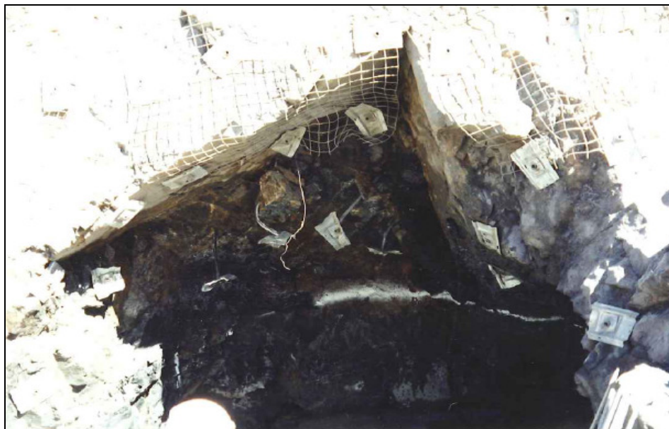
Figure 2.7 Wedge fall from roof near the portal of an excavation
