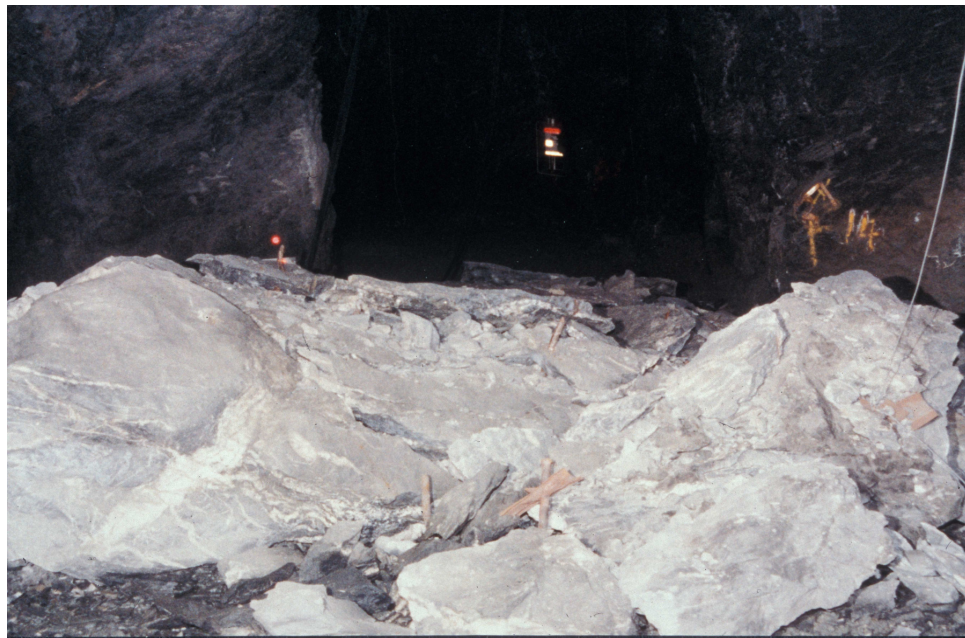
Figure 2.14 Gravity induced rock slab failure
