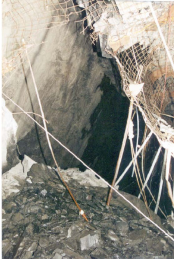
Figure 2.11 A prism failure from the roof of an excavation
