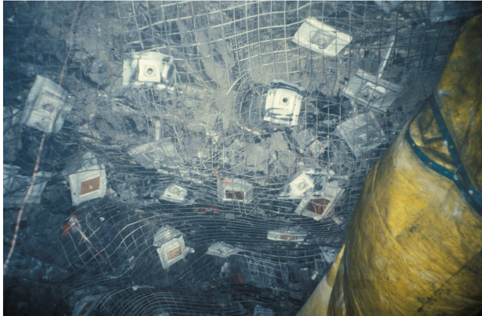
Figure 2.20 Spalling rock in the roof held by mesh
