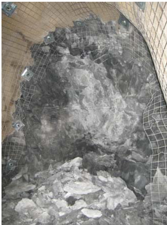
Figure 2.19 Strain burst damage on the excavation face
