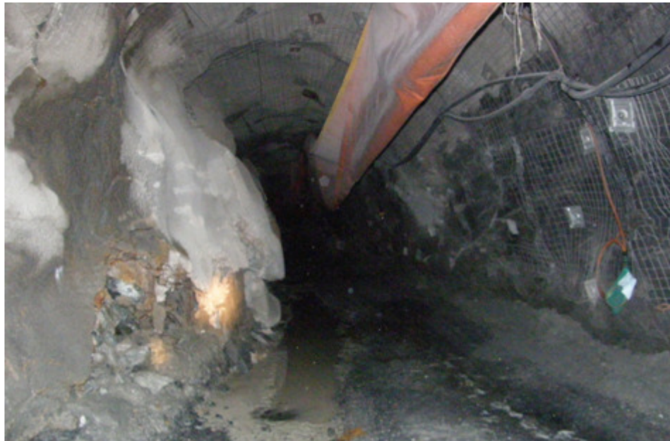
Figure 2.22 Squeezing rock on left wall
