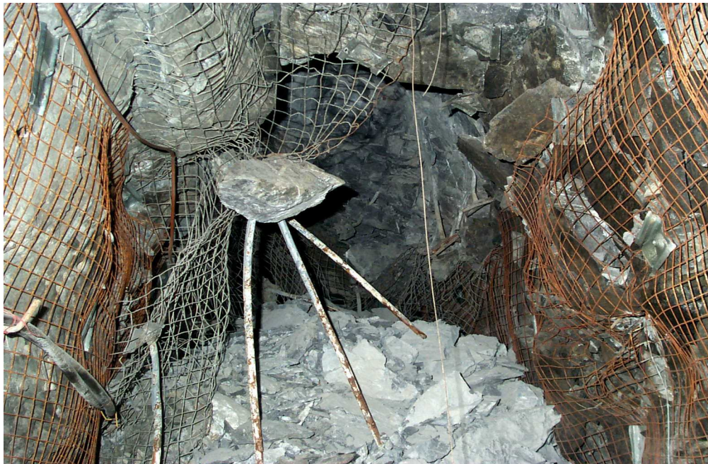
Figure 2.24 Unravelling in heavily jointed rock in a intermediate stress conditions
