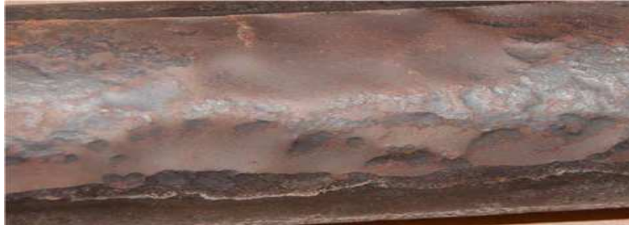
Figure 2.5 Eroded tube surface
