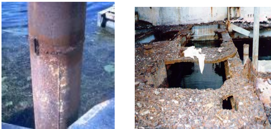
Figure 2.21: Uniform corrosion of structural steel (KSC, 2009)
