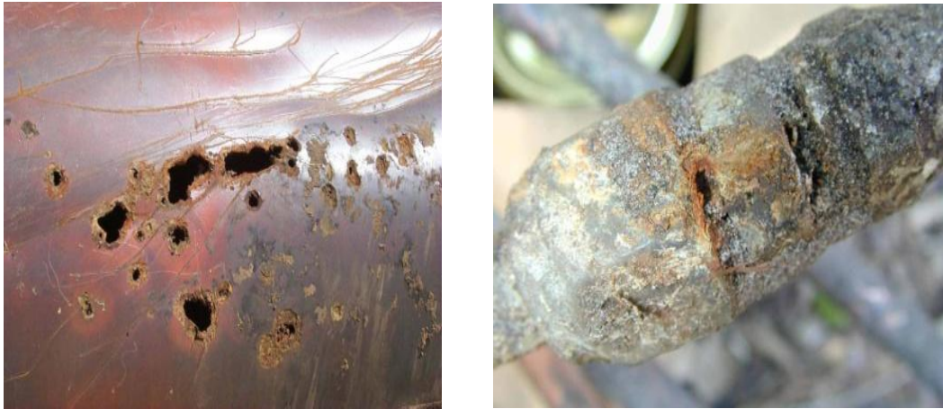
Figure 2.16: Metals attacked by galvanic corrosion (Obanijesu et al, 2010c)
