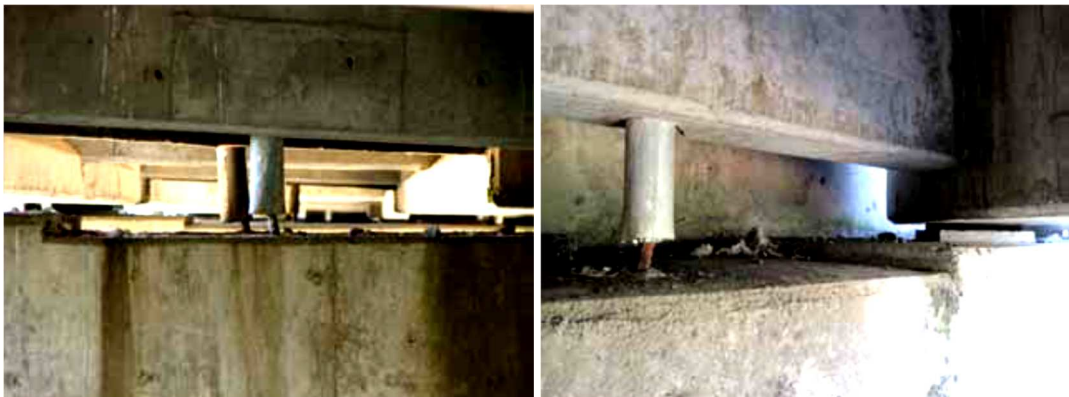
Figure 2-7 Metallic yielding dampers on Chilean bridges (Elnashai et al., 2010).
