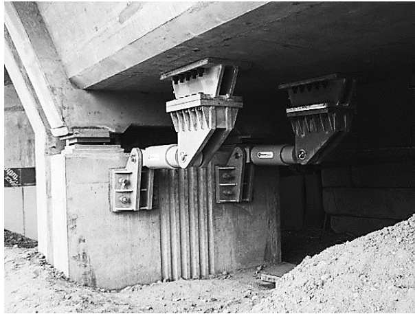
Figure 2-12 Shock transmission unit installed in a bridge.
