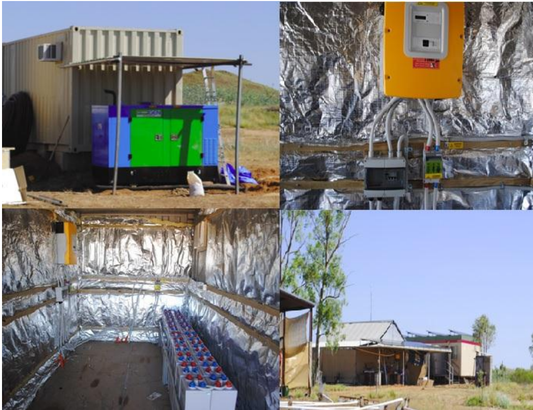
Figure 4. 25: System after installation and commissioning
