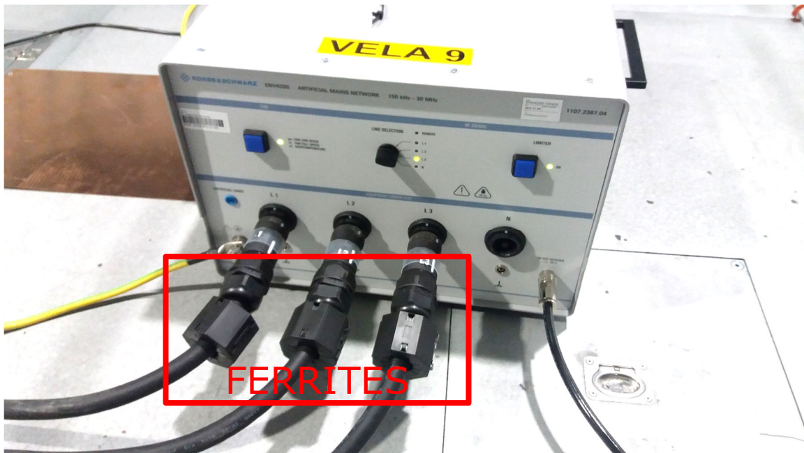
Figure 51: Charger 'C' installation of clamp-on ferrites to investigate their effectiveness on the suppression of the conducted emissions. Thick wires go towards the HPC column.
