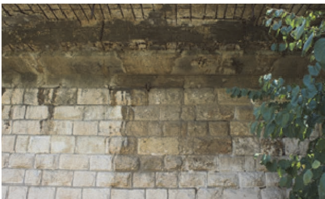
Figure 4. Bulging and colour change at the spandrel wall
