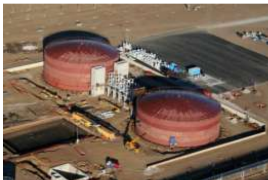
Fig.1. Andosol 3 Thermal storage tanks
