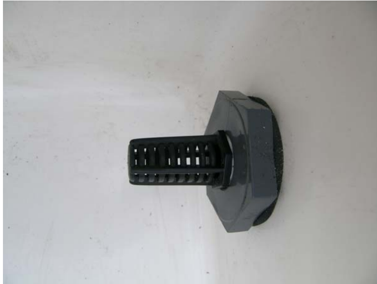
Figure 9: Tidal Exchange plumbing (interior) with no standpipe.
