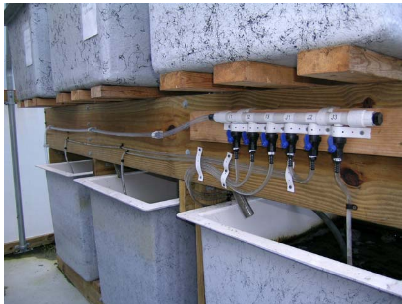
Figure 29: Air distribution gang valve
