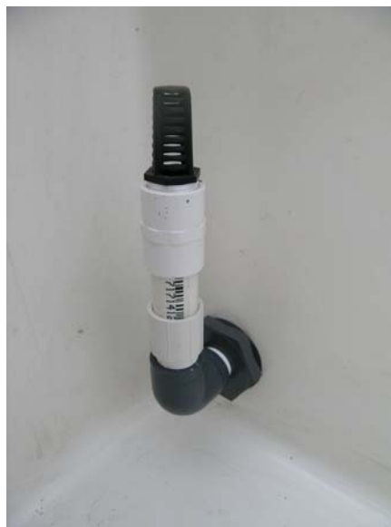
Figure 8: Tidal Exchange plumbing (interior standpipe) assembled
