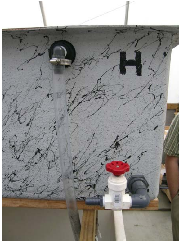
Figure 12: Completed mesocosm plumbing for upper tank
