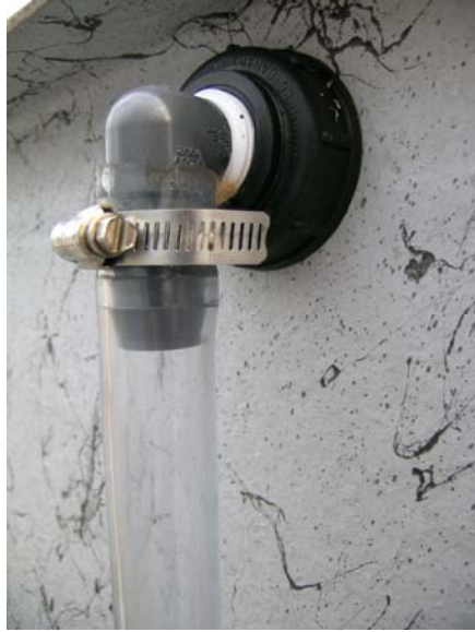
Figure 10: Overflow plumbing (exterior)
