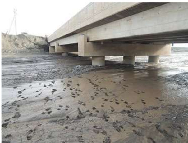
Figure 1. Thick sediment deposition in Gobu River at the small town of Waja.
