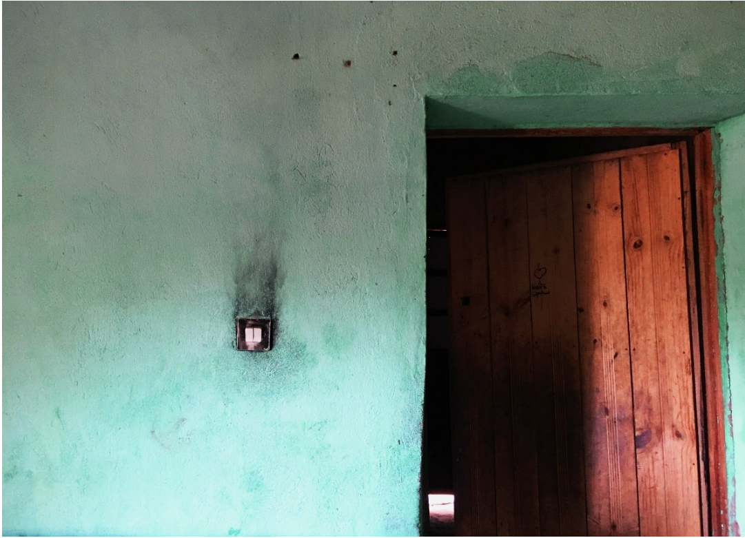
Figure 5.80. A switch in PPW15 participant’s house which burnt having experience a short electrical circuit. Photo credit: I. Bisaga.
