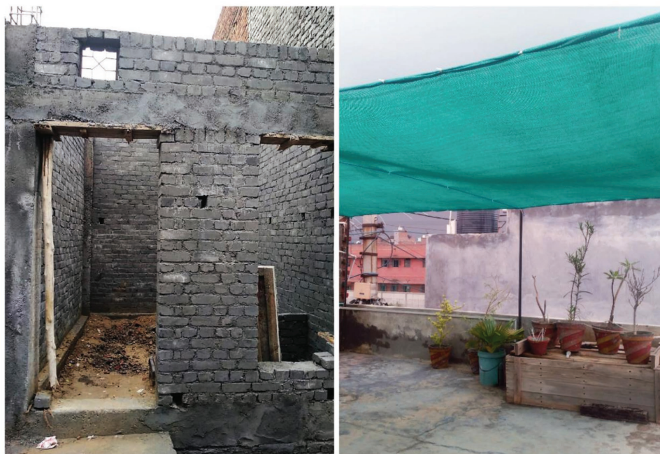
Figure 5. On-going construction of a newly designed house (left) and implemented solar shading on an existing roof (right).
