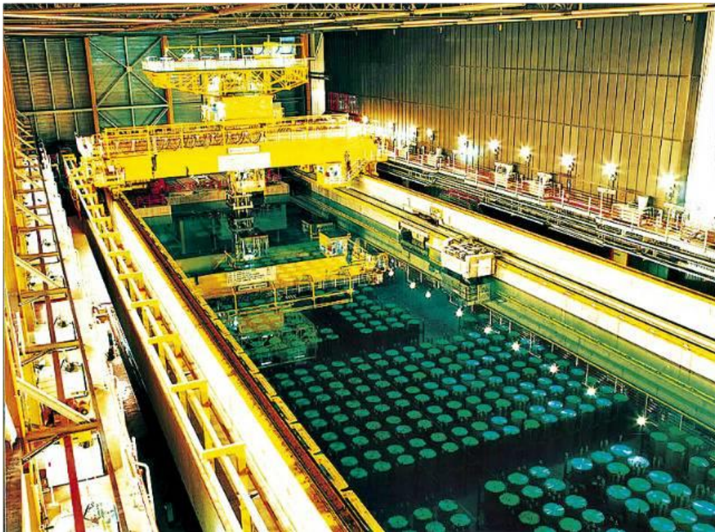
Figure 1.11 – Cooling pond of the Thermal Oxide Reprocessing Plant (THORP) at Sellafield site [50].
