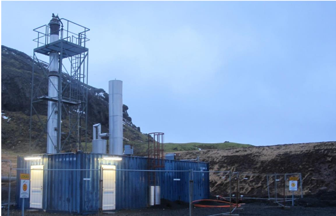
Fig. 4. The pilot gas capture plant, with the scrubber tower (right), deaerator (lowest column in the middle) and the distillation column, the tallest column on the left (Photo: Ingvi Gunnarsson).
