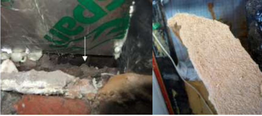
Figure 5. (left) and 6 (right) Illustrates a blocked airbrick, unintentionally caused by placing rigid insulation boards between the joists. Figure 6. illustrates chamfering of the insulation to aid instead of obstruct airbrick airflow.
