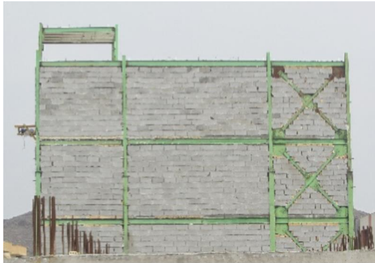
Figure 5.5 - Side view of the index building (No stair case elevator core is built for the Index building)
