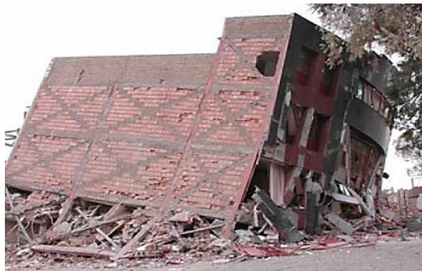
Figure 1.4 – Soft storey failure of masonry infilled steel frame, observed during 2003 Bam earthquake (Manafpour, 2003)
