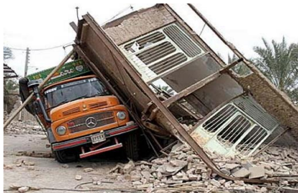
Figure 1.3 - Cases of heavy damage and collapse due to connection and masonry infill wall failure, observed during 2003 Bam earthquake (Manafpour, 2003)
