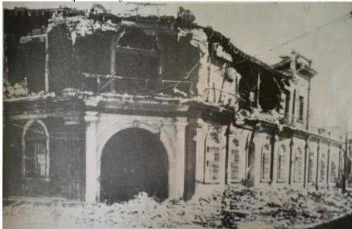
Figure 5-26 Damage to the electrical company building during the 1912-3 earthquake sequence, from Taracena Flores (1970)
