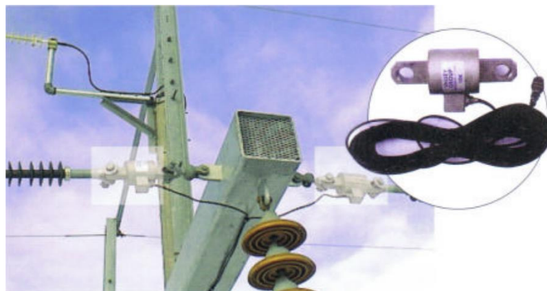
Fig. 2-17. Load cells mounted between the cross arm of a strain structure and insulators [59]
