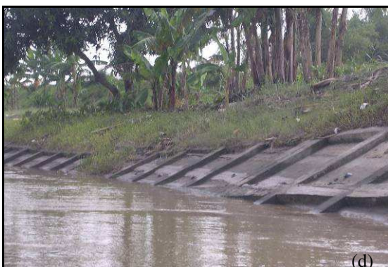
Fig. 2. Failures along the Bengawan Solo Embankments: (a) erosion of natural embankments; (b) shallow failure of man-made embankment; (c) global failure of gabion reinforced embankments; (d) differential settlement under concrete protection slabs.
