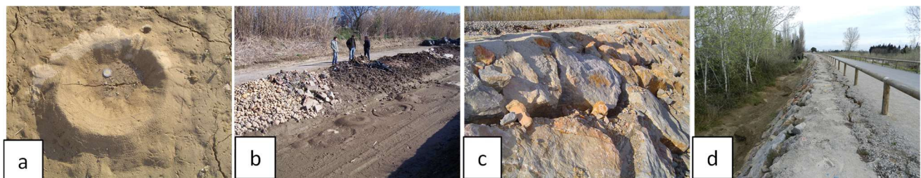
Figure 13. a) Sand boil (photo: Pierre Philippe, CEMAGREF), b) Multiple sand boils close to the maintenance track on the landward side of the dike (photo: Patrice Mériaux, CEMAGREF), c) Damage to the dike itself: cracks on the crest and in the riprap landside revetment (photo: Pierre Philippe, CEMAGREF), d) Damage to the dike itself: crack on the crest; this picture was taken in 2013 but similar damage occurred in 2006 (photo: Patrice Mériaux, Irstea).
