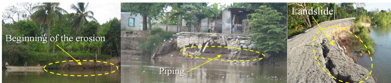
Figure 4. Evidence of instability in river banks and dikes induced by rapid drawdown in Villahermosa.
