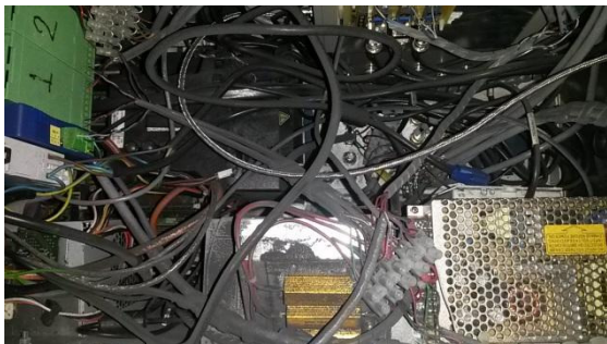
Figure 1: Large volume of dust inside enclosure
