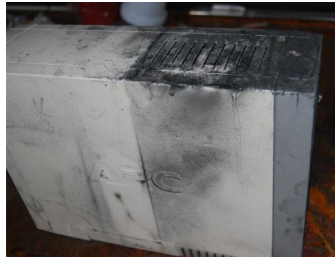
Figure 2: Failed UPS due to excessive dust
