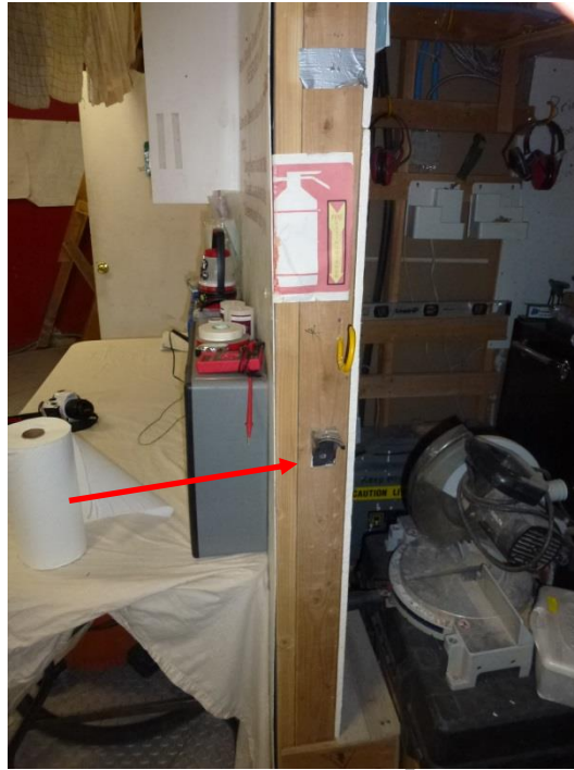
Figure 5 Damaged fire extinguisher bracket on the MDRS
