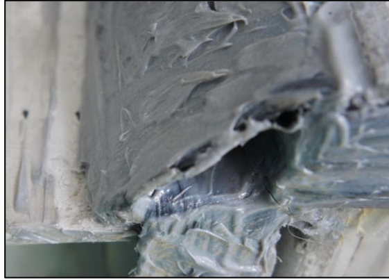
Figure 7. BTCj_fcrww: slip between “closed” seat angle and the upper flange of the beam.
