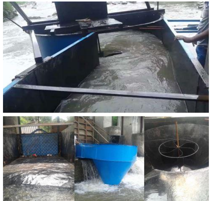
Fig. 16: Pilot Project using conical basin structure (canal, gate, basin structure and runner)
