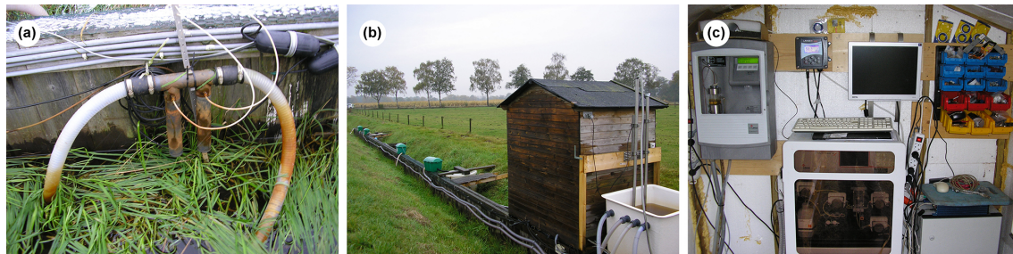
Figure 3. Pictures of the controlled drainage period setup: (a) the drainage overflow levels were adjusted by attaching the flexible connection tube (with a SorbiCell socket between the black fasteners) at the desired level; (b) the tube drain effluent was pumped to a collection vessel to enable continuous monitoring of \text{NO}_3\text{-N} and total-P concentrations using a Nitratax-UV sensor and a Phosphax auto-analyzer (c).
