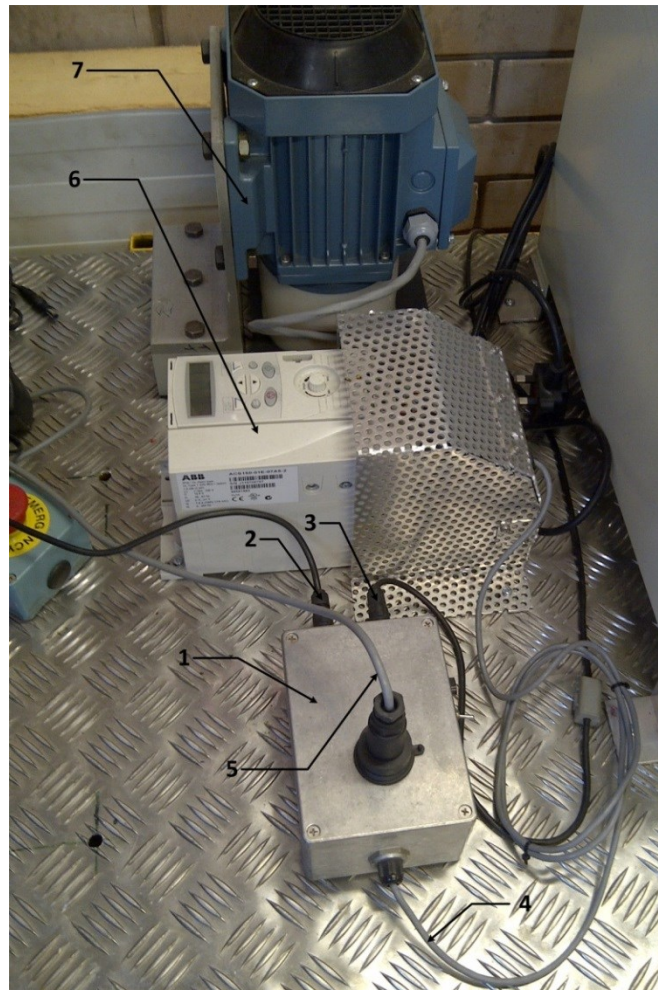
Figure 3.10 Illustration of the motion controller agent and its components. Labels: 1→ Developed position/speed controller, 2→ position feedback signal from odometer, 3→ RS232 serial I/O port, 4→ Analogue output, 5→ emergency stop signal, 6→ ABB VFD inverter, 7→ three-phase AC motor used to propel the trolley.
