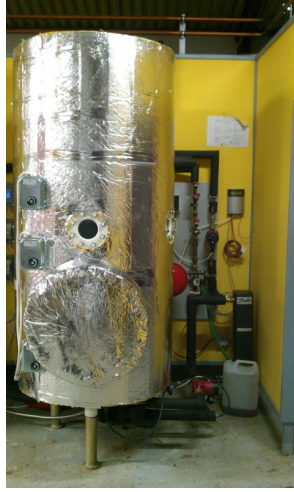
Figure 2.3: Heat storage tank connected to solar thermal collector on building roof.
